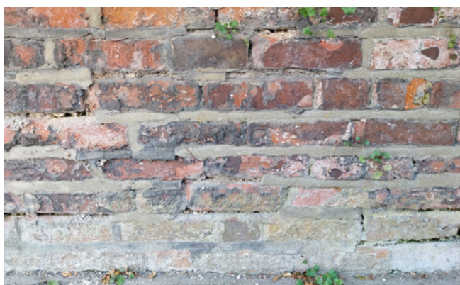
Poorly executed cement mortar repointing
