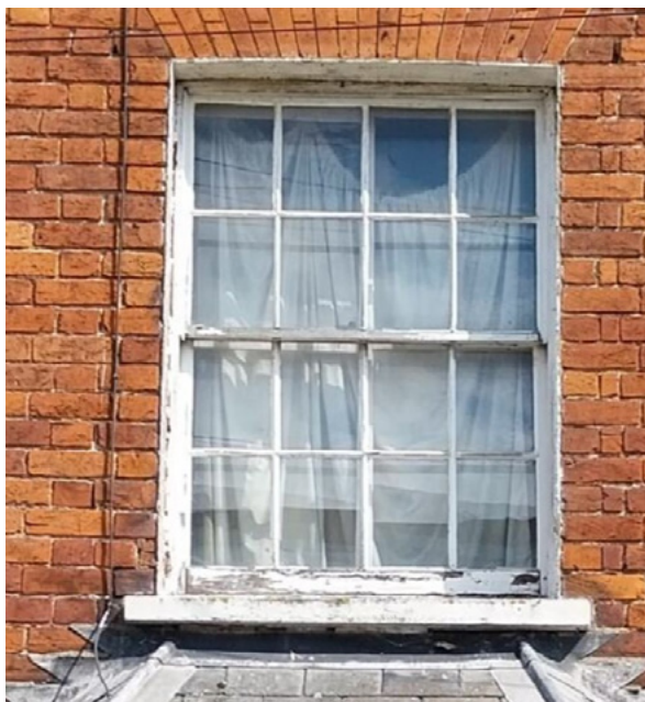
Peeling paintwork on an historic timber window
