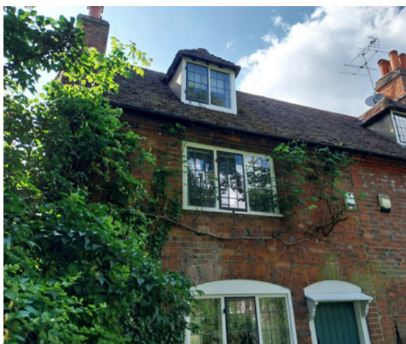
Invasive ivy growth can damage masonry
