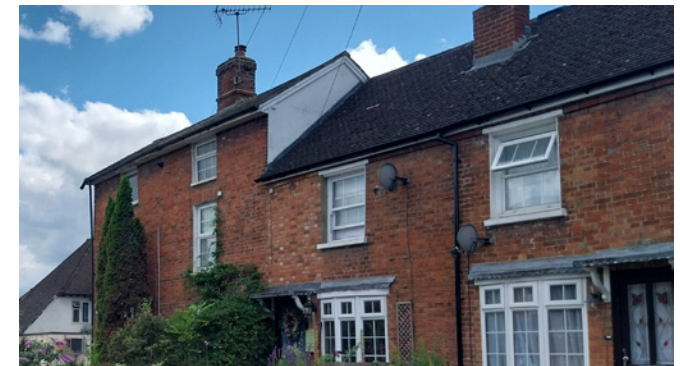
Satellite dishes, aerials and electric wires add detritus to building frontages
