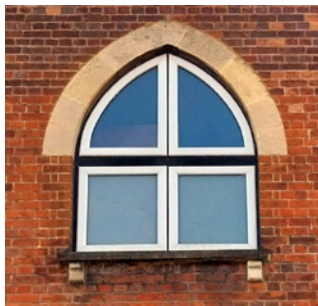
Inappropriate uPVC windows
