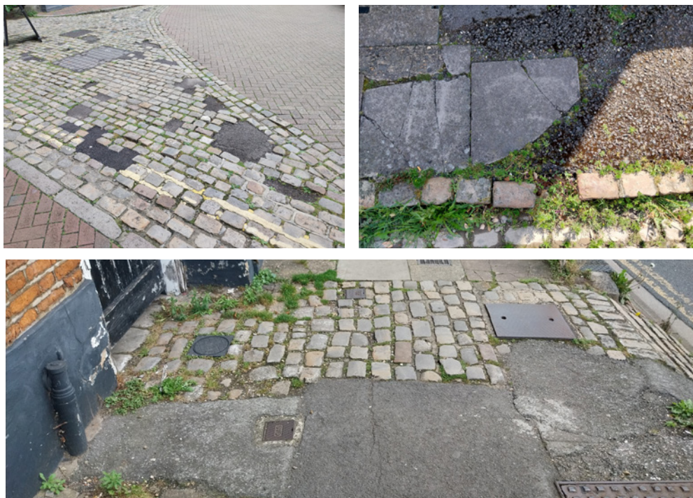
Pavements scars are common across the Conservation Area and detract from its appearance
