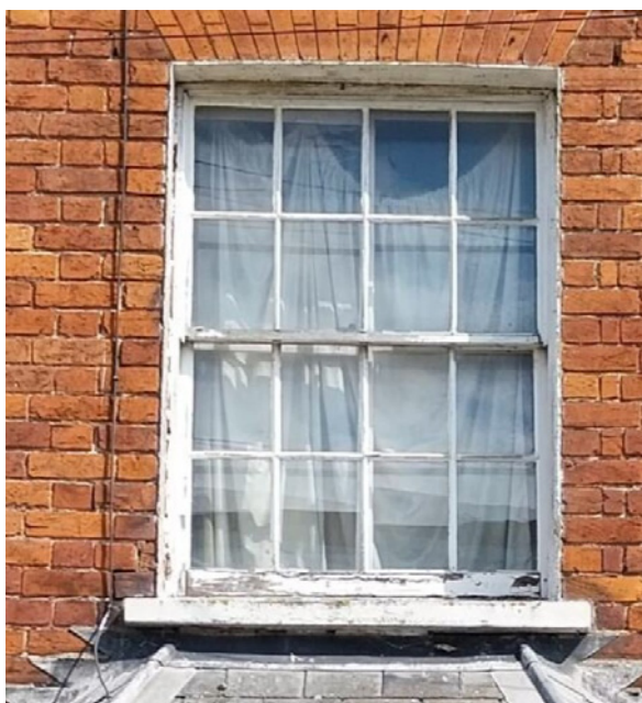
Peeling paintwork on an historic timber window
