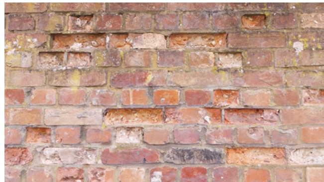
Brick that has worn away due to moisture being trapped within the wall because of cement mortar pointing
