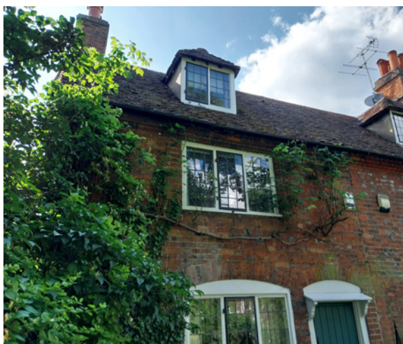
Invasive ivy growth can damage masonry
