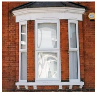
Inappropriate uPVC windows
