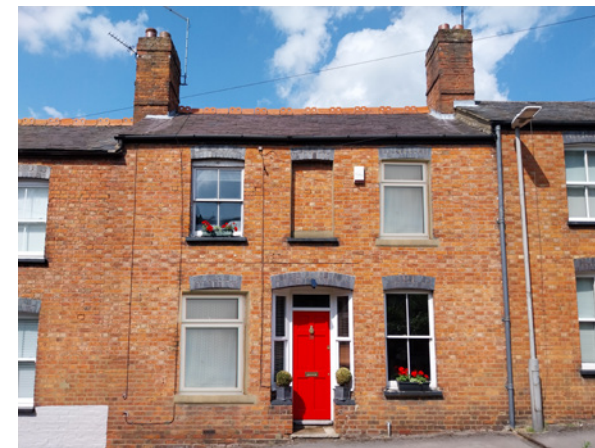
The piecemeal insertion of uPVC windows, which do not follow the traditional glazing pattern and require the widening of openings, skew the proportions of details such as window headers and the symmetry of the building.
