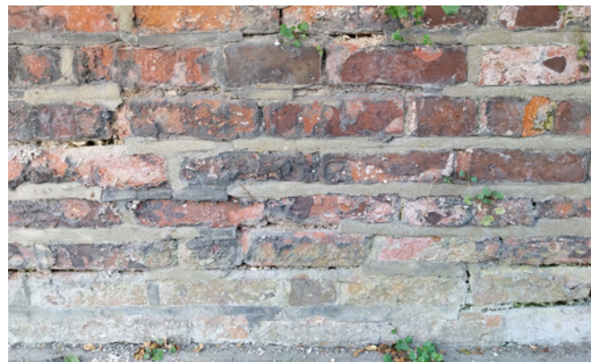
Poorly executed cement mortar repointing
