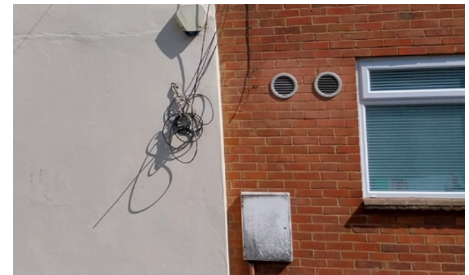
Loose wires and service boxes
