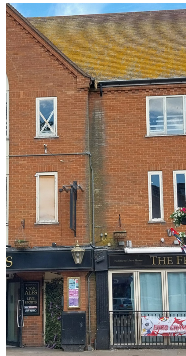
Discolored masonry from rainwater overflow and lichen on roof tiles
