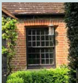
Dark walnut timber sash window
